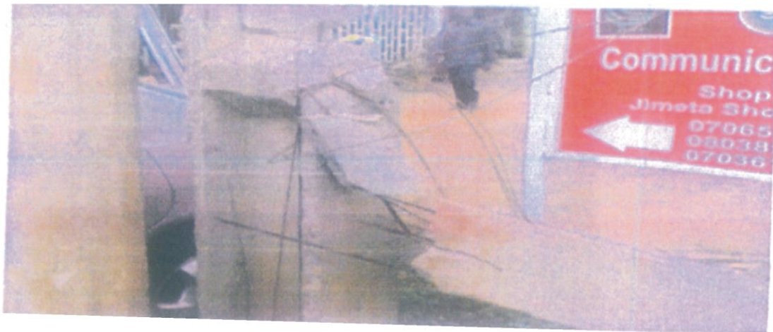
Plate I: Failure of Reinforced Concrete Pole with 12mm bars at Jimeta Shopping Complex
