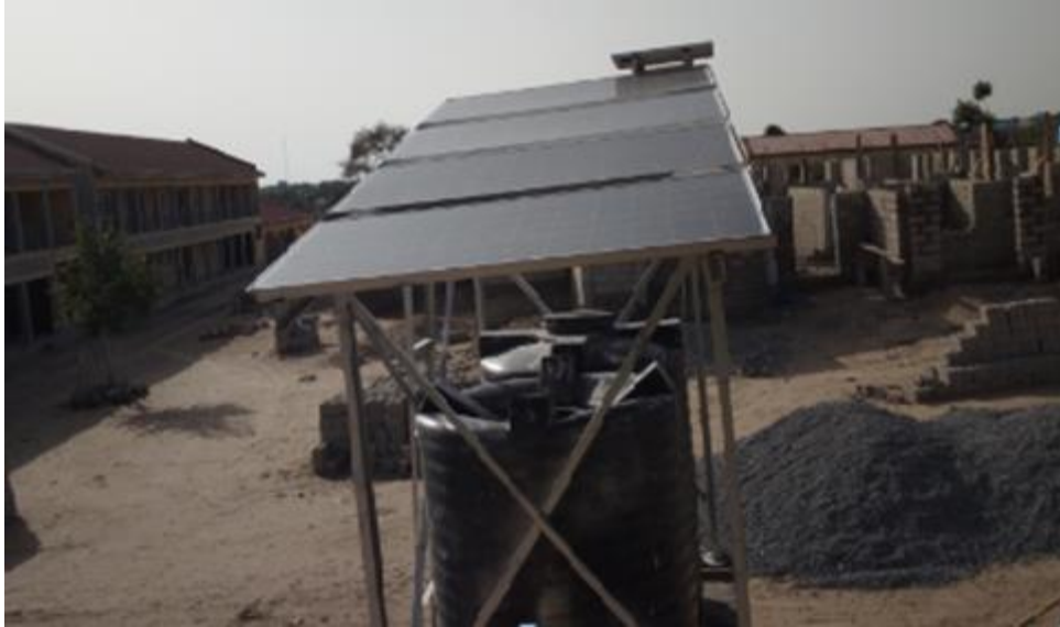
Figure 1. PV modules of 310 W each, installed in parallel and constituting the photovoltaic panel system installed at the Galtimari Primary School Jere Local Government, Borno State, Nigeria.
