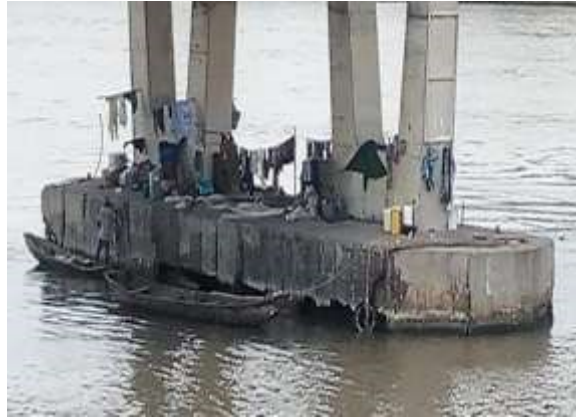
Plate 1. A spalled section of a Pile cap in a beach environment in Lagos, Nigeria
